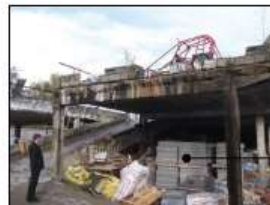
VIEW E - SHOWING HEIGHT OF EXISTING STRUCTURE AND CENTRAL RAMP AT REAR.
