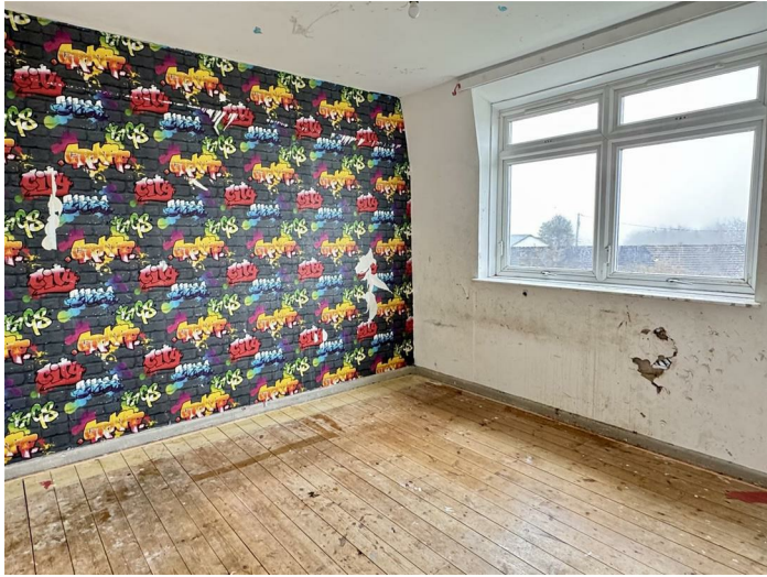
Upvc double glazed window to the front elevation. Door provides access to inbuilt storage void. Wall mounted Dimplex Quantum electric heater. Exposed wood flooring.
