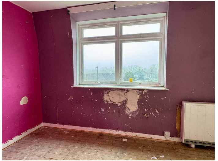
Upvc double glazed window to front elevation. Airing cupboard housing the unvented pressurised hot water cylinder. Exposed wood flooring, Wall mounted Dimplex Quantum electric heater.
